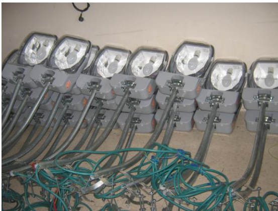
Street lights, Al-Walajeh.
