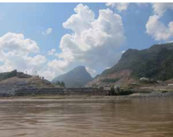
The site of the Xayaburi dam at the beginning of its construction in 2012. The dam is nearly half complete, according to the Thai firm tasked with its construction. https://www.flickr.com/photos/internationalrivers/8159583340/
