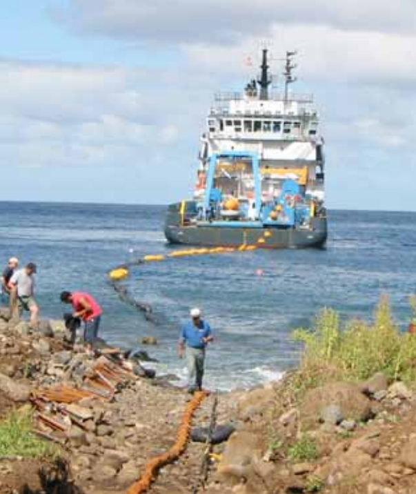
Installing the underwater cable of hydroacoustic station HA03, Juan Fernandez Island, Chile, in 2003.
