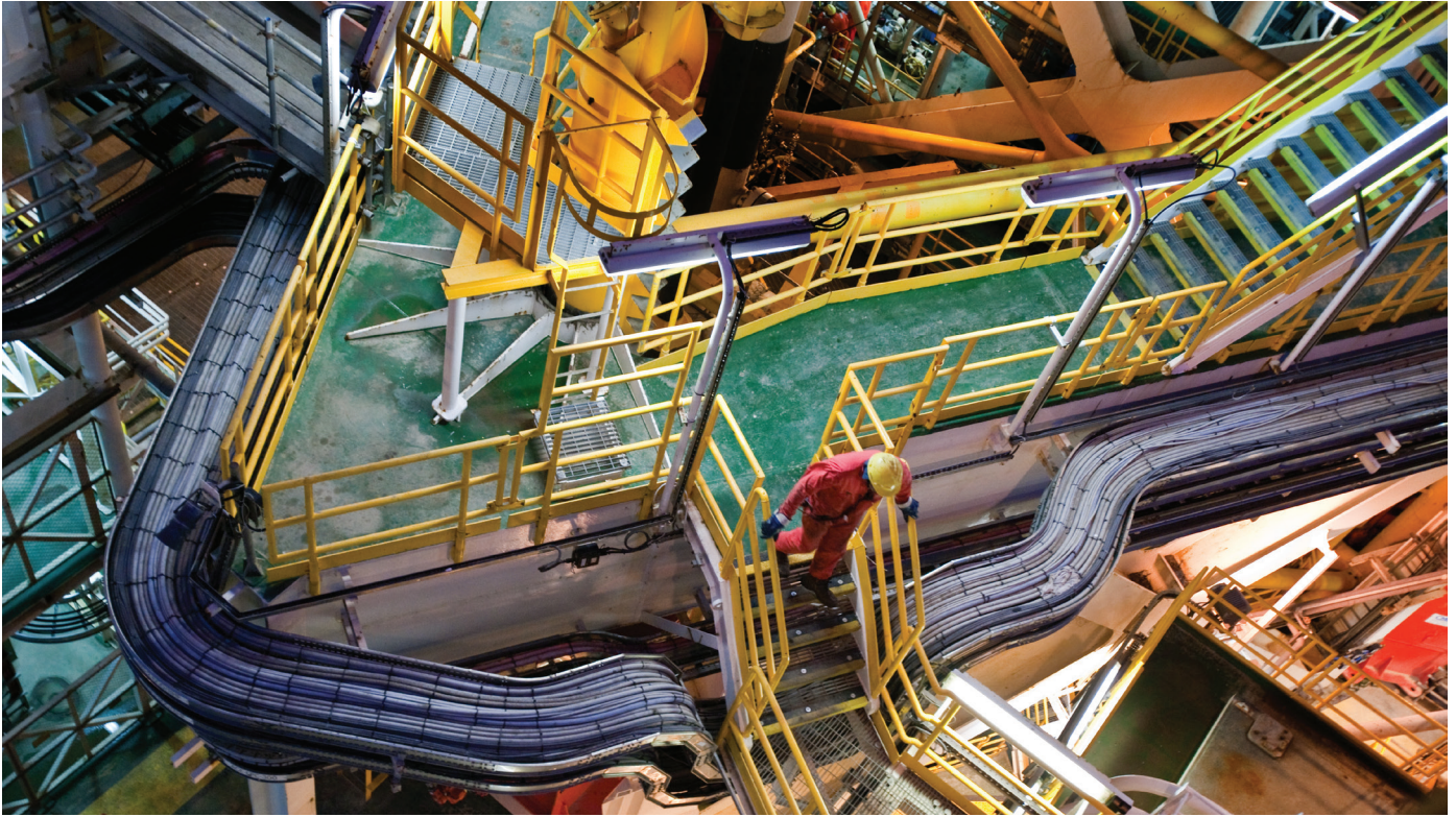
A worker on a BP Platform in the Shah Deniz gas field, Caspian Sea
