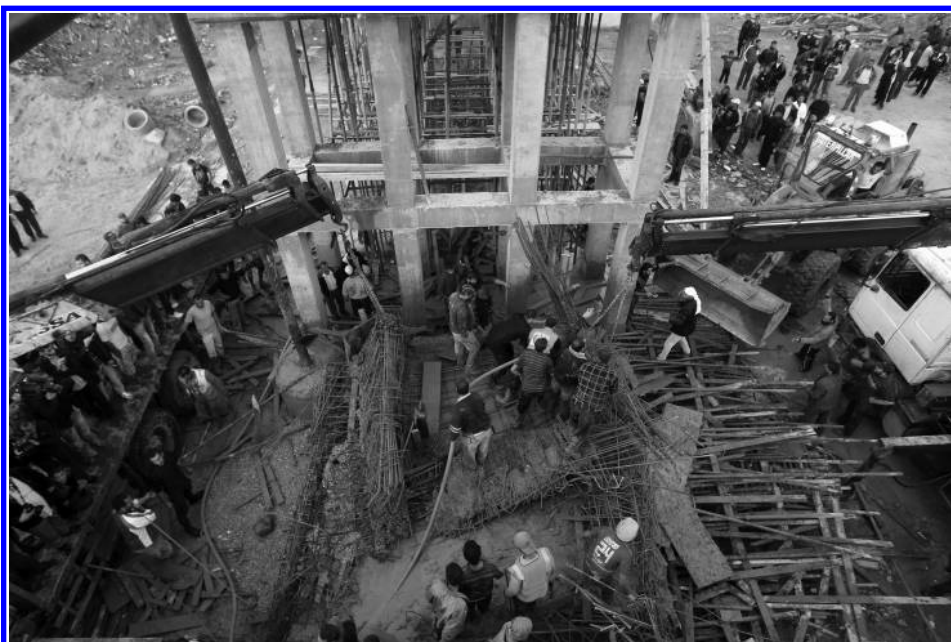
Palestinian rescue teams inspect the scene of a collapsed bridge on a main road near Nussayrat linking Gaza City with the south, 17 November 2011. One Palestinian worker was killed and five others were wounded when the bridge collapsed. (Mohammed Abed/AFP/Getty Images)
