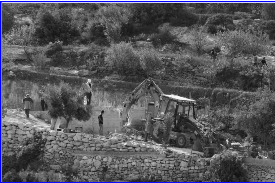
An Israeli tractor demolishes a Palestinian water well in the West Bank village of Bayt Kahil, on the outskirts of Hebron, on 6 October 2011. (Hazem Bader/AFP/Getty Images)
